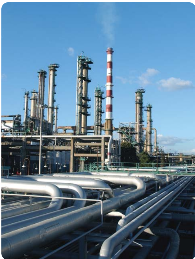
Aromatics plant at Oporto refinery
